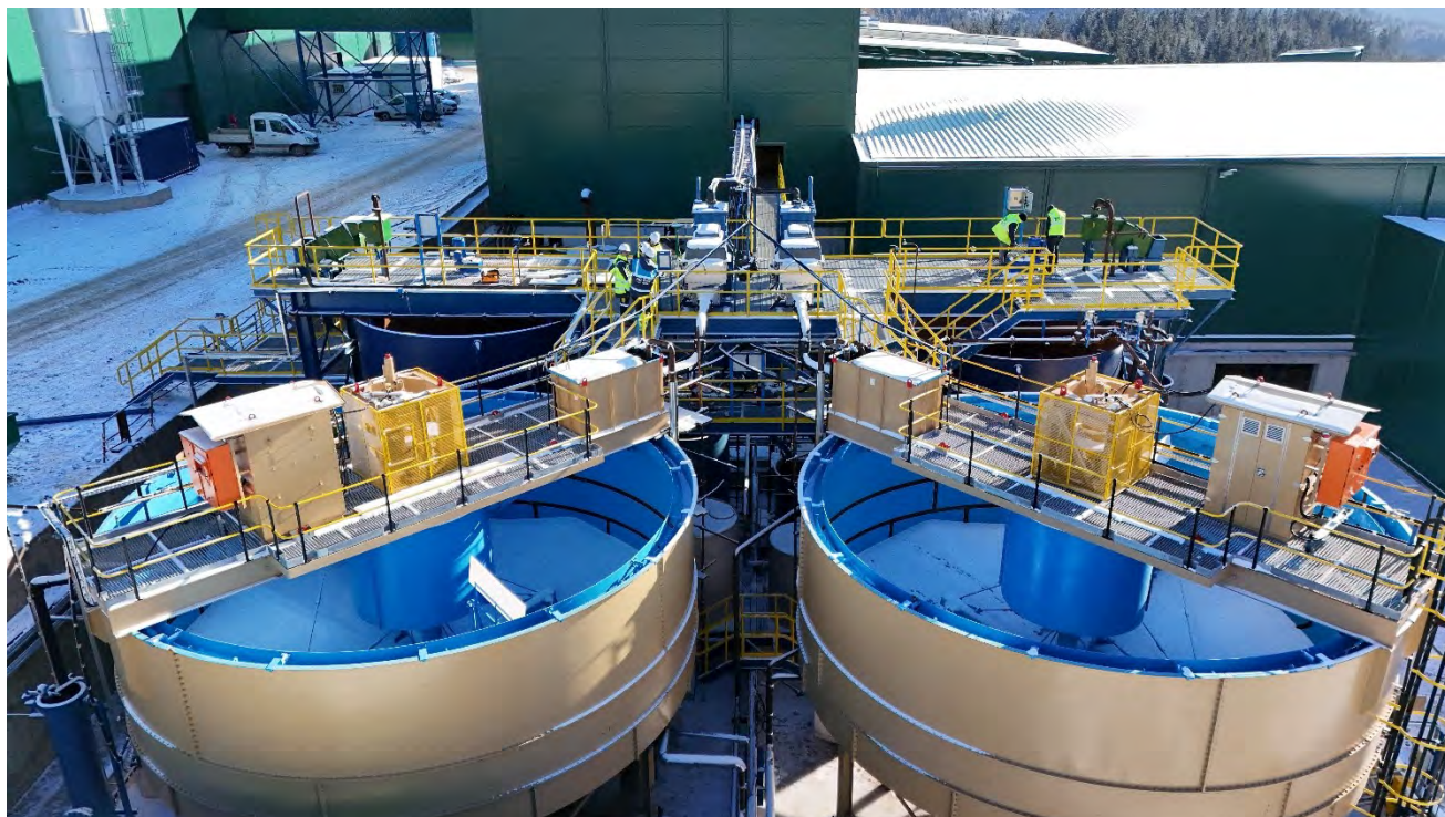
Figure 12: Thickeners (lead and zinc), January 2024
